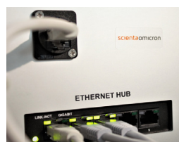
Ethernet Rack Upgrade
