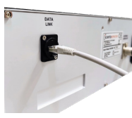
Ethernet Rack Upgrade
